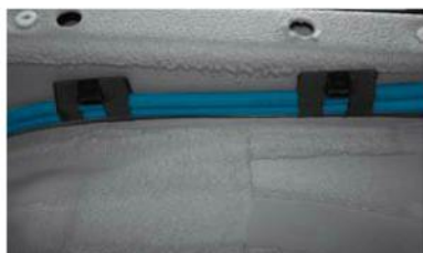
Figure 18.7 Câbles haute tension.
